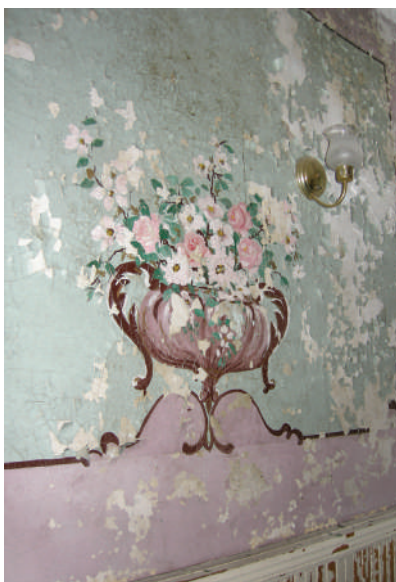
23. Downstairs Community room - Scheme 3 - only murals to remain uncovered since date of painting
